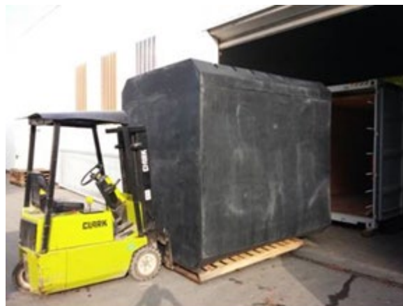
denitrification installation into a sea container
